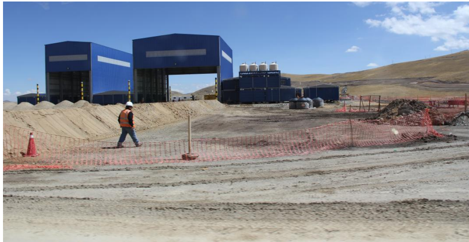
Constancia mine maintenance facilities
