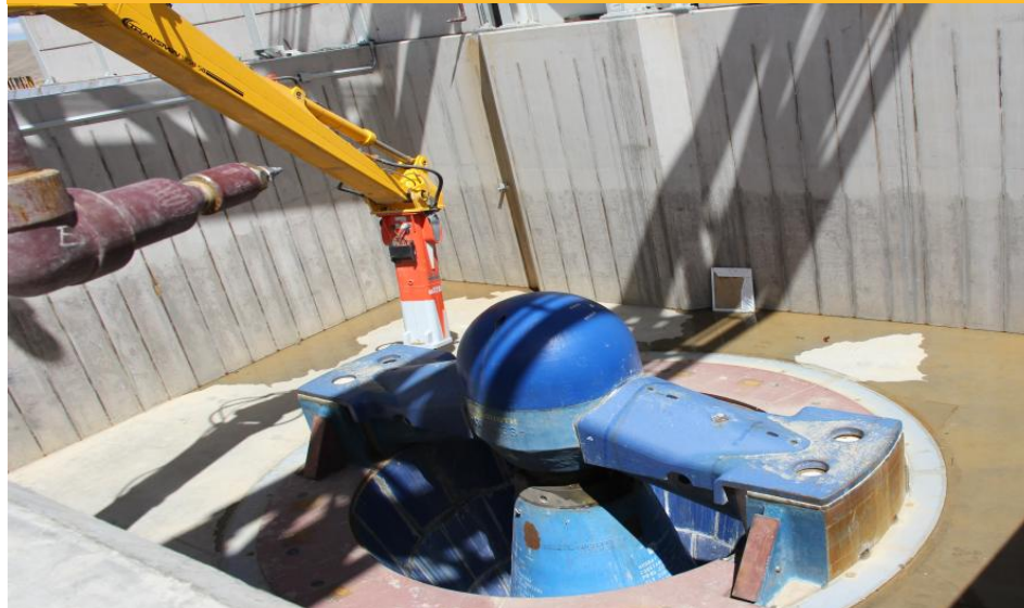
Constancia ore dump pocket for the primary crusher
